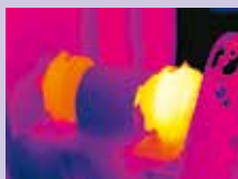
Overheating bearing cap
